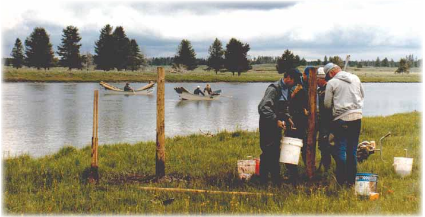
Volunteers from the Henrys Fork Foundation helped put up barbed wire fence in 1986. Eight miles of the Henrys Fork are fenced on both sides of the river to keep cattle out of the river, protect streambanks and fish habitat. Ranchers and HFF are responsible for maintaining the fences, even before cattle are in the park in the fall.
