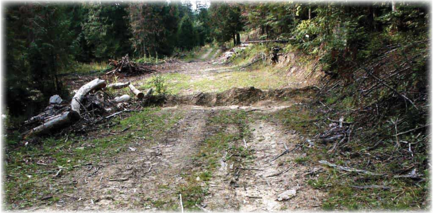
Water bars, also known as cross ditches are used to drain water across forest roads.
