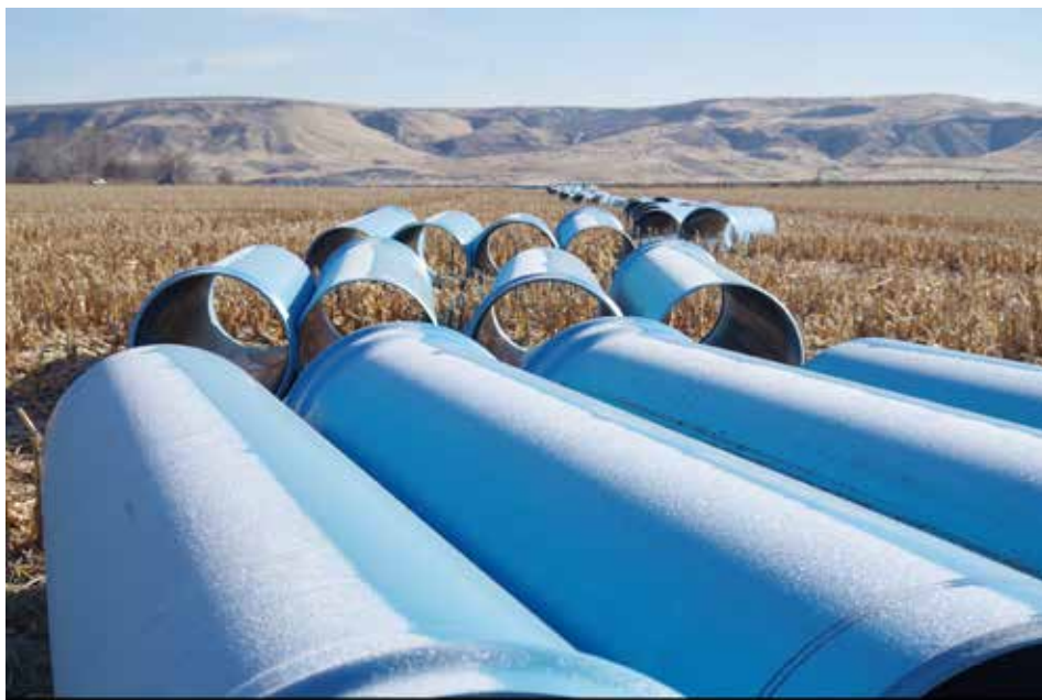
LEFT: About five miles of irrigation pipeline was buried by the Snake River to reach about 120 different farms and water users spread over 2,000 acres of land.
