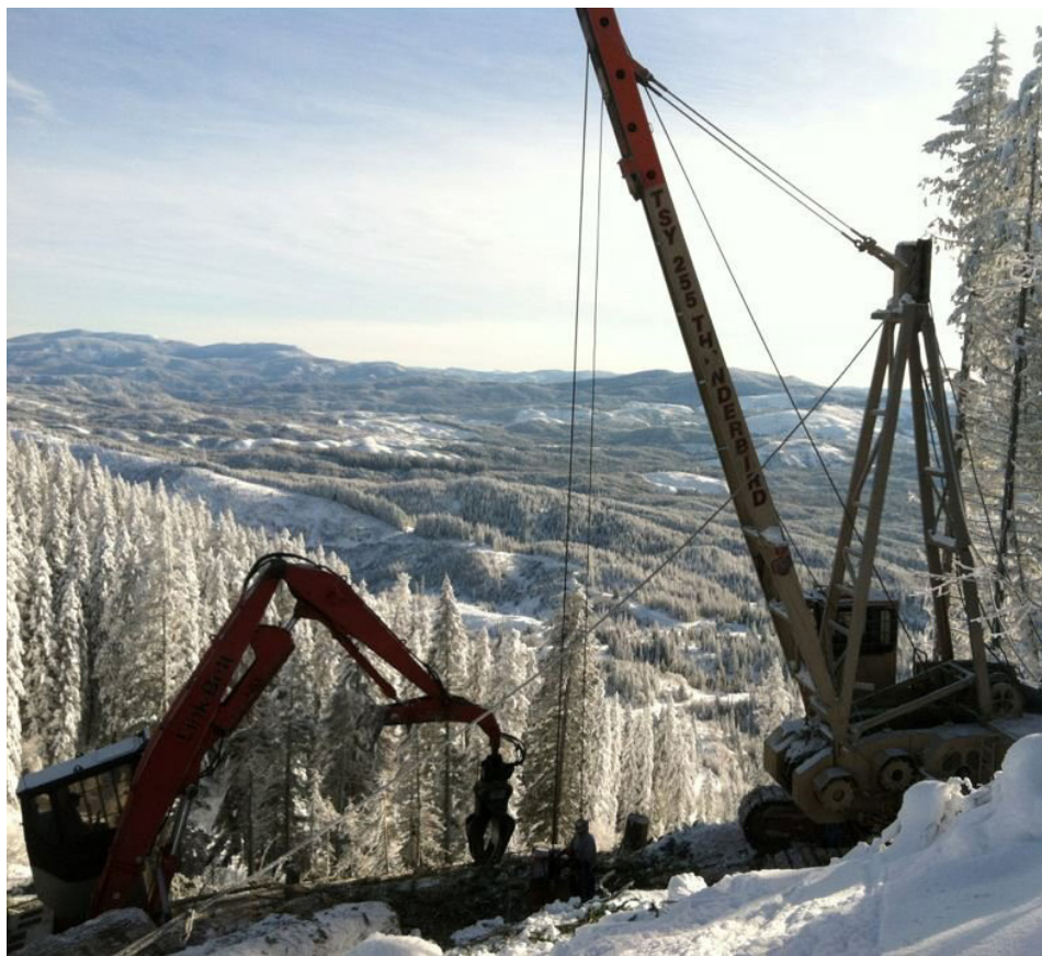
Cable yarding with a Thunderbird line machine is used in areas with steep slopes. A loader for loading logs on trucks sets to the left of the line machine.
