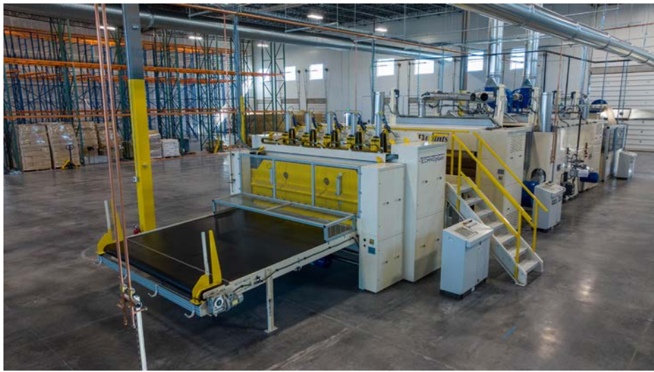
Hempitecture's new manufacturing facility in Jerome, shown here, uses about 36,000 pounds of industrial hemp every two weeks.
